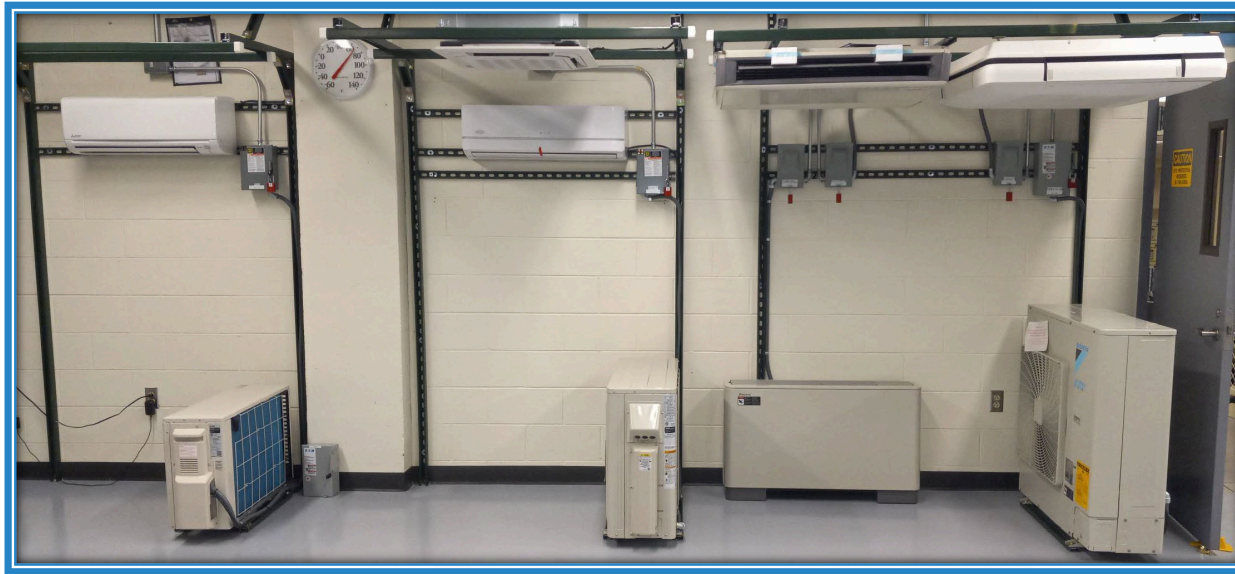
Heat Pumps & Mini Splits Training
